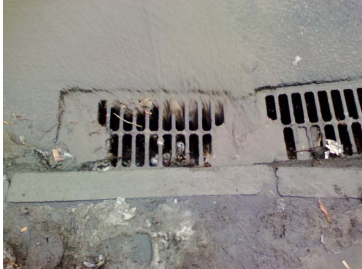
Polluted water runs into a storm drain.
